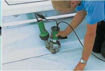
TRIAC DRIVE PID used for welding plastic roofing membranes in a light dome.
