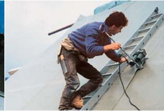
X84 used to weld an under-roof liner on a high-pitched roof. Weighing only 6.1 kg, the X84 copes with any incline at constant speed.
